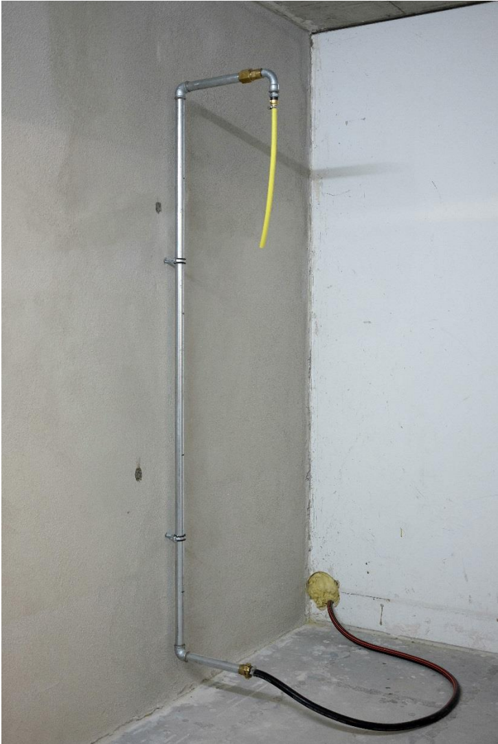
Figure 2: fresh water pipe attached to the installation wall
